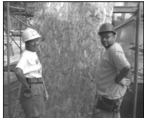
Linda Heffernan and Fred Black rest from working on the Building Hope Partnership home.
