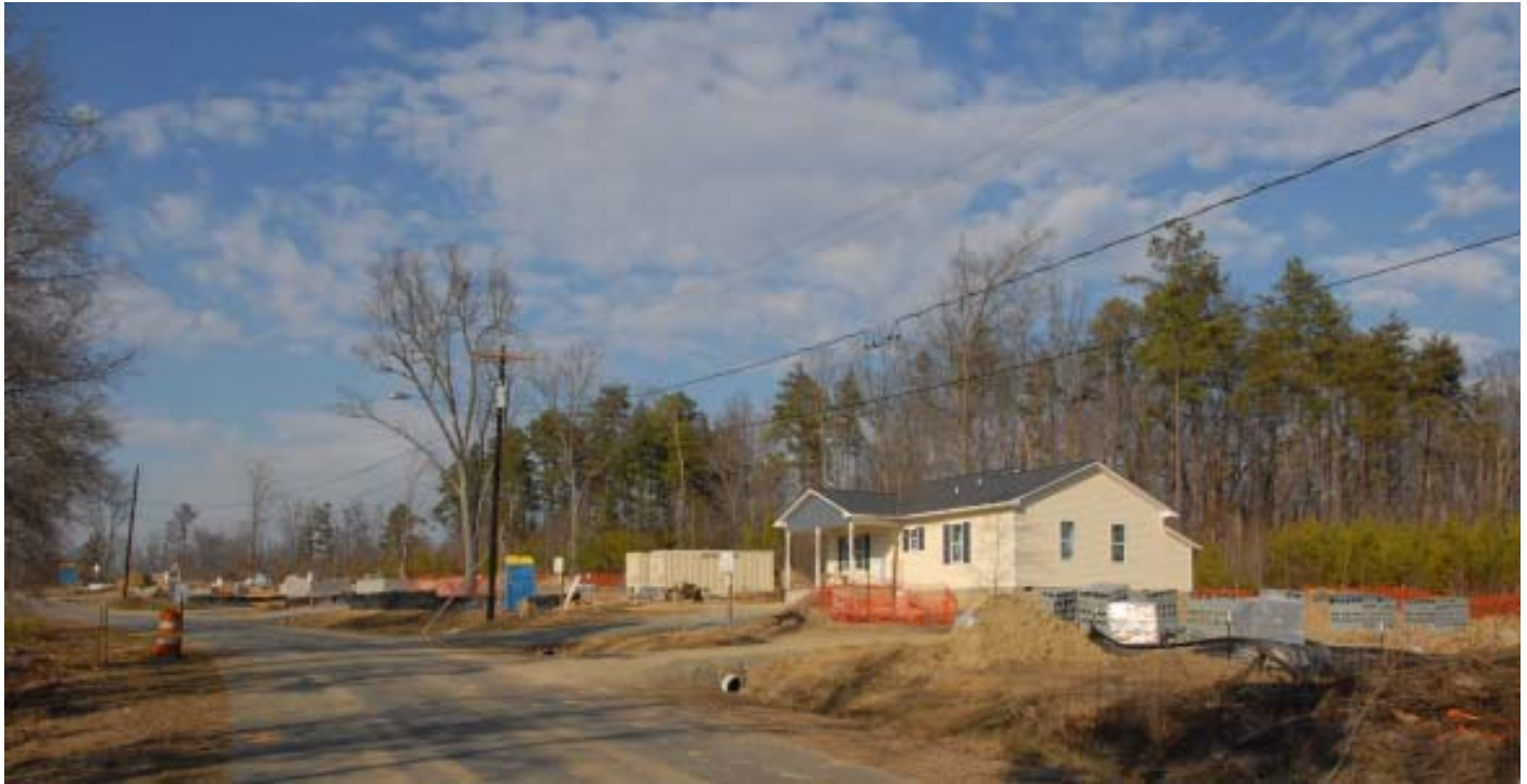
Tulip Tree Road in Hillsborough's Fairview community is a happening place these days. Habitat will soon complete the first home, the second home has been blitzed (see page 6) and foundations are in place for three more homes.
